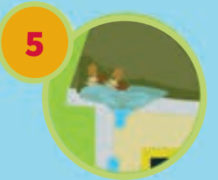
5 Clogged rain gutter.
